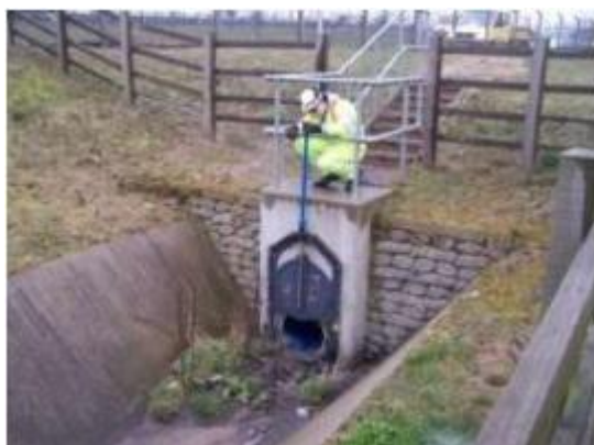
Sluice valve Photo courtesy of Carillion-URS
